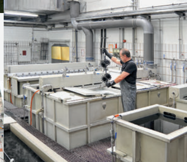
Manuell bediente Eloxalanlage Manually operated anodizing plant
